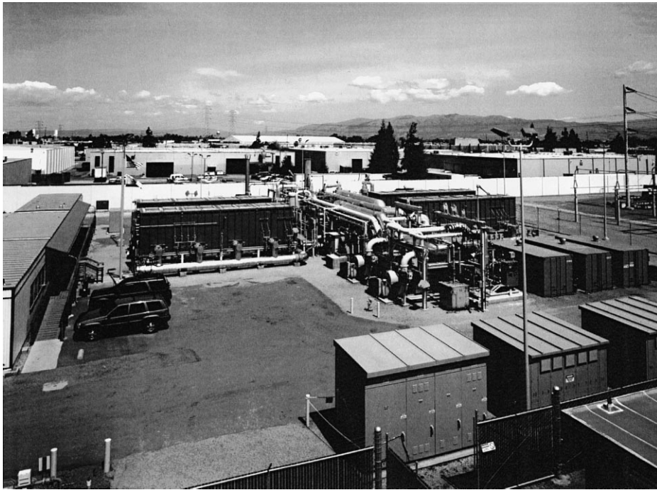
Fig. 6. Direct Fuel Cell™ power plant demonstration at Santa Clara, CA.
